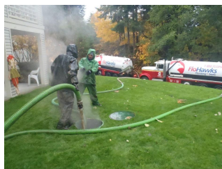
Back flushing to break up the scum layer is intense aerosolization of liquids with no eye or respiratory protection with humidity and cool weather shows how much aerosolization is occurring.
